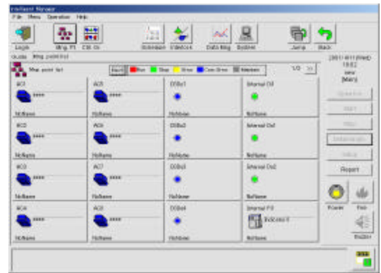
Monitoring PC (on site)
